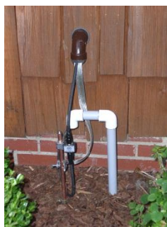
Shack end - Ground Rod and PolyPhaser protection
